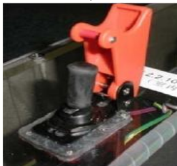
紧急断开 Emergency disconnection
